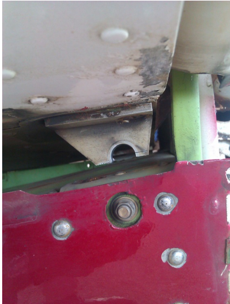
Cessna 200 series horizontal stabiliser attachment bracket fatigue failure
